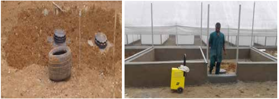
Figure 15. Left picture are tanks of 1000 l buried and right is the mason work of the power house.
